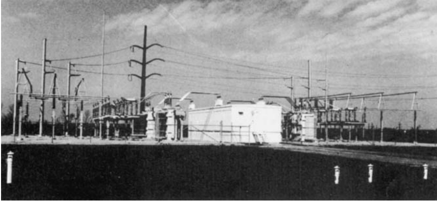
FIGURE 4.116 Installed power-distributing center for a brewery in the northeastern United States.
