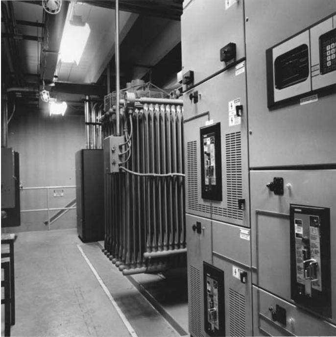
FIGURE 5.11 Liquid filled transformer utilizing silicone liquid listed by UL as a dielectric medium and less flammable per 450.23 of the NEC. [Dow Corning]
