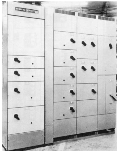
FIGURE 4.122 Power-control-center switchboard. [General Electric Co.]
