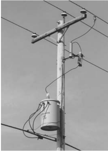
FIGURE 5.78 Pole-mounted 30-kVA distribution transformer protected with conventional surge arrester and separate current-limiting fuse. [Cooper Power Systems]
