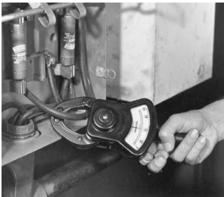
FIGURE 1.72 Application of Tong-Test ammeter. [Martindale Electric Co.]
